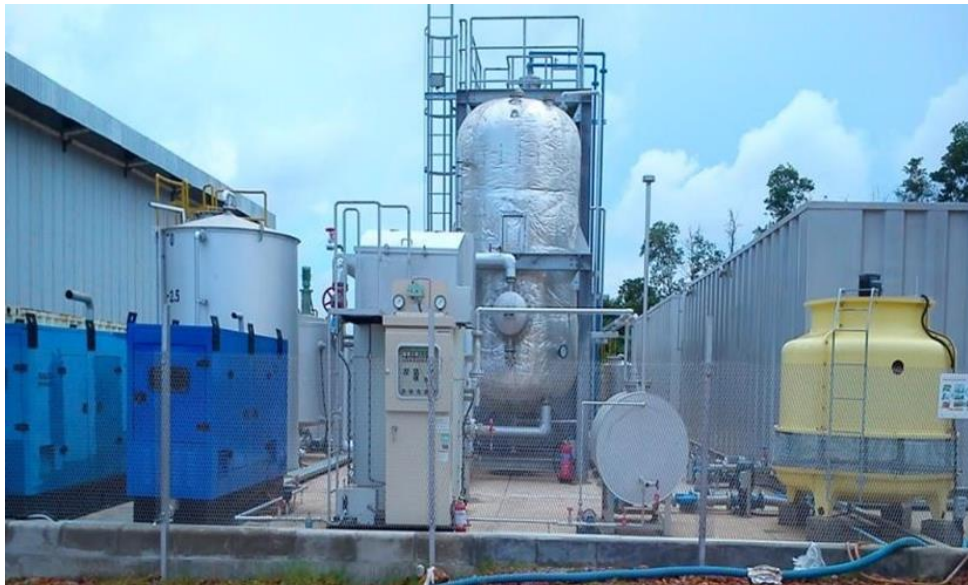
Figure 5. Demo of used lubricating oil processing plant into MFO
