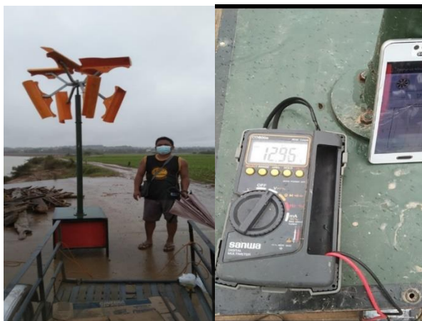
Figure 17. Testing of the Vertical Axis Wind Turbine
